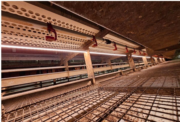
AVIARY-LIGHT installed under the multi-tier system.
