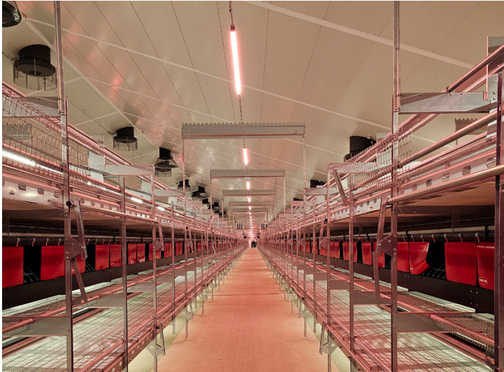
Ceiling lighting installed in a layer house with a multi-tier system.
